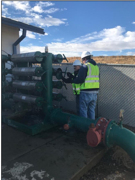
Water treatment plant employees performing winterization on pivot feed line filters.
