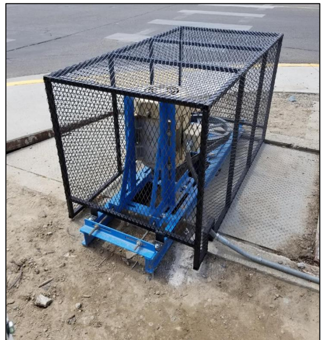
Bottom: New protective cage for Verde Irrigation Pump.
