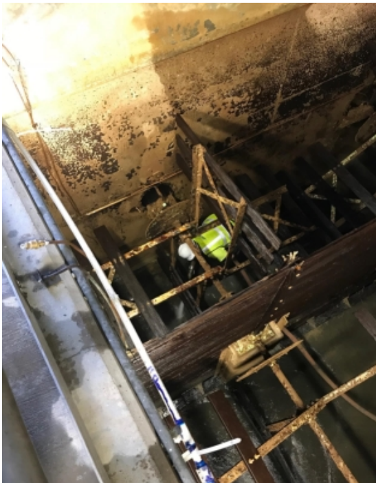
Cleaning flocculation basin
