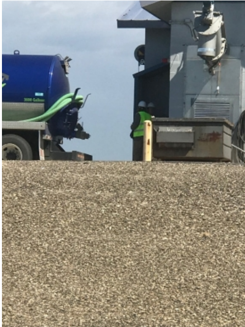
Receiving septage load
