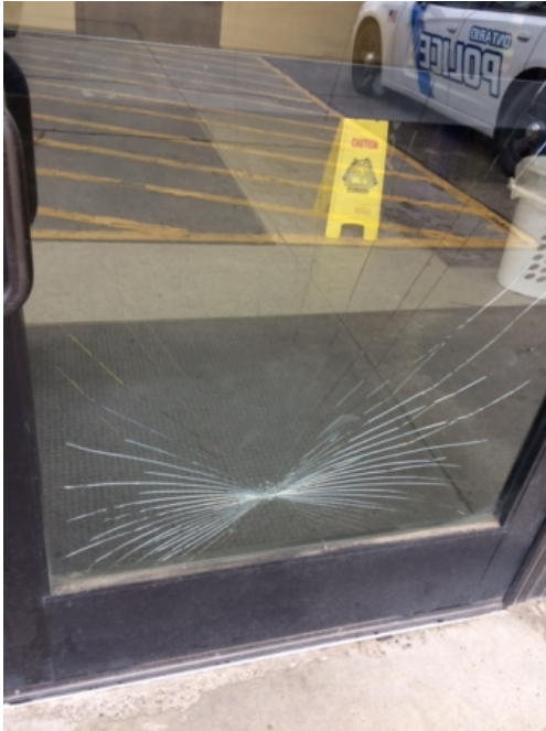
Broken glass on backdoor at City Hall
