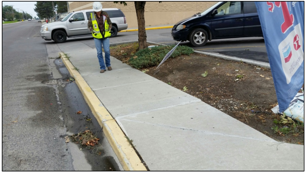
CH2M engineering technician inspects sidewalk pumping along Alameda Drive after several trip and fall complaints. Property owner hired a private contractor to pump up the low spots on the sidewalk and eliminated the uneven panels.
