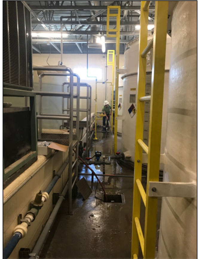
Water Treatment Plant employee performing routine housekeeping at the WesTech Plant.
