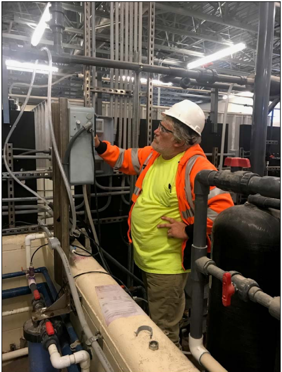
Water Treatment Plant employee calibrating water quality instrumentation.
