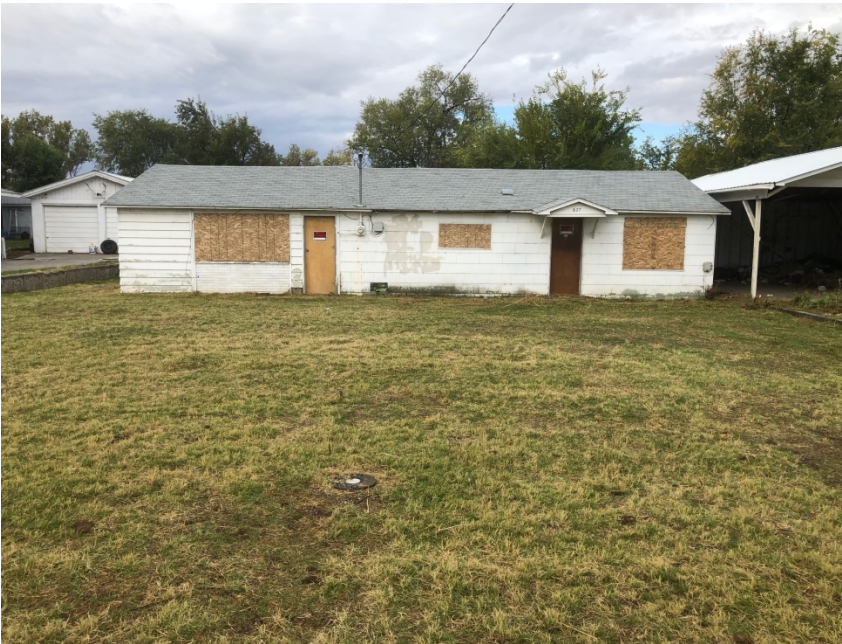
627 Fortner St – Derelict Structure & Weeds/Garbage & Transient Issues
