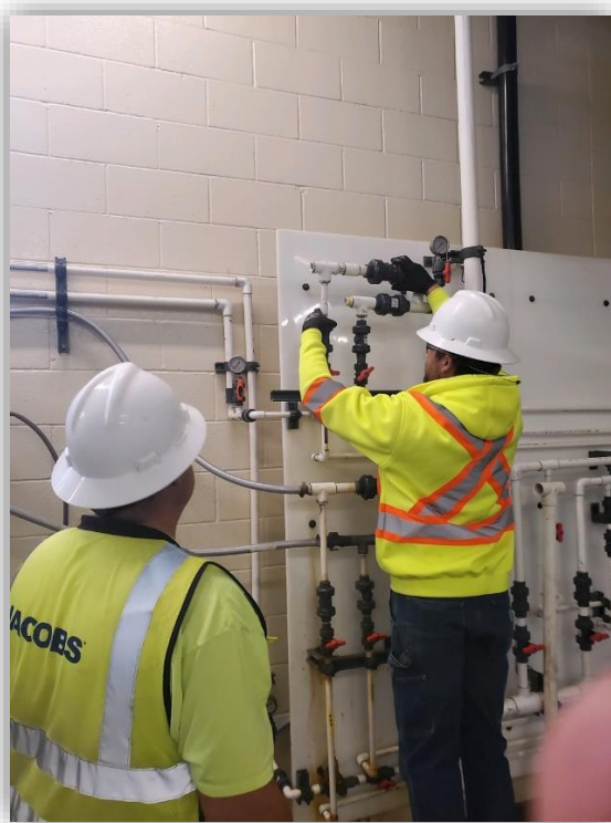
Above: Jacobs staff performing maintenance on \text{Kmno}_4 chemical feed line.
