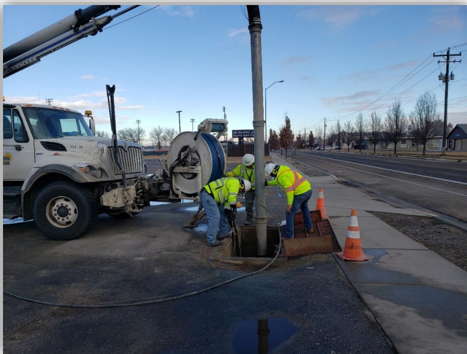
Above: Jacobs crew cleaning Storm water line at TVCC with our jet rodding equipment
