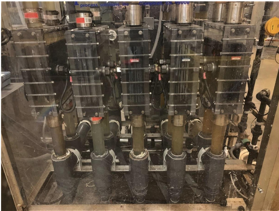
MicroChlor chlorine generator cells after being cleaned and acid. washed
