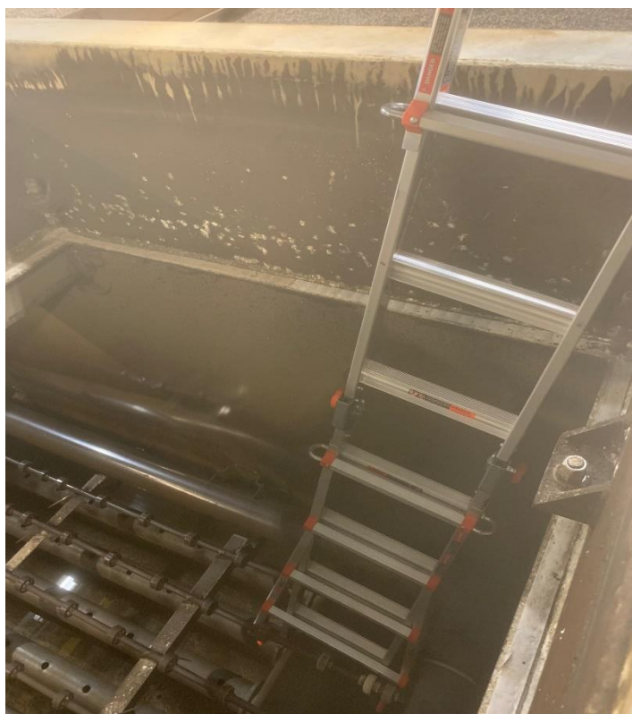
Below: Annual maintenance on WesTech clarifier #1.
