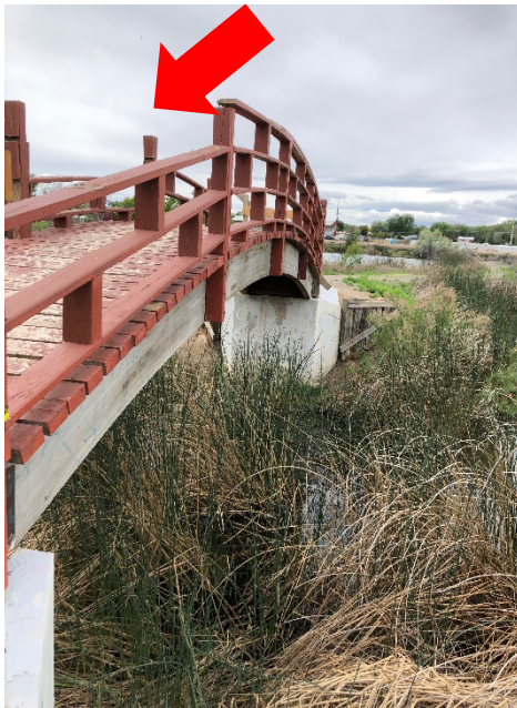
More rail damage
