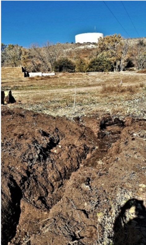
Bench Reservoir over-flow piping
