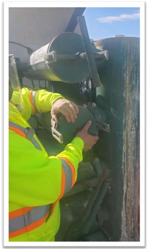
Performing maintenance on "Everfelt" filter system at skyline farm.
