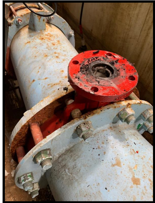
Above: Filter #2 Effluent Valve Removed for Service.
