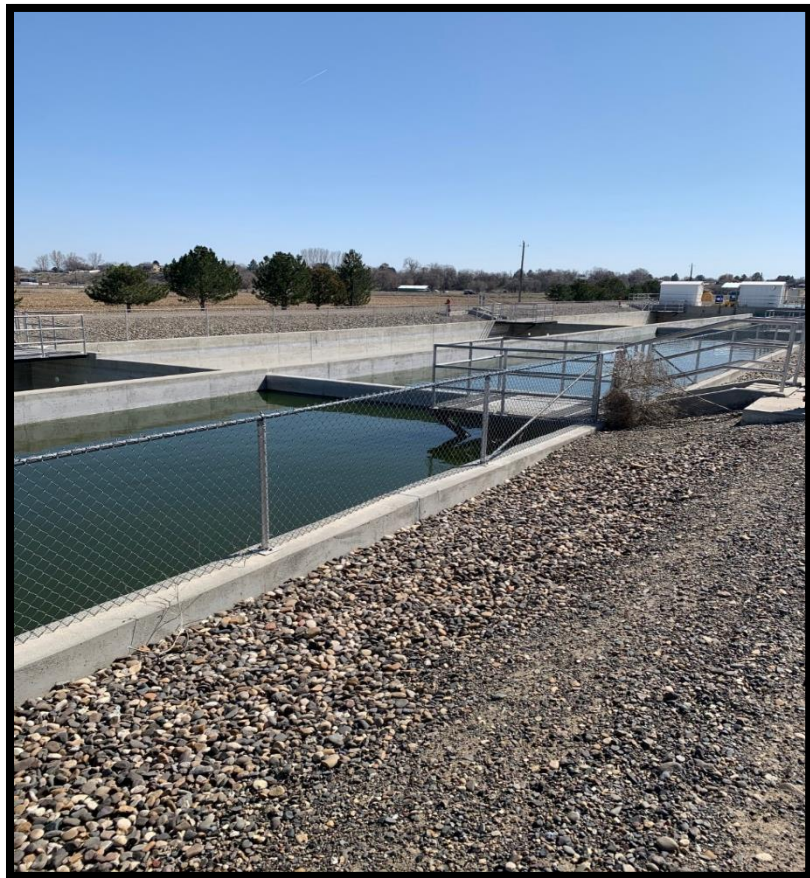
Chlorine Contact Chambers at WWTP
