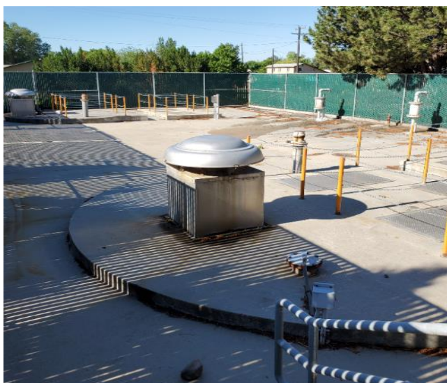
NW 8 th Ave Lift Station
