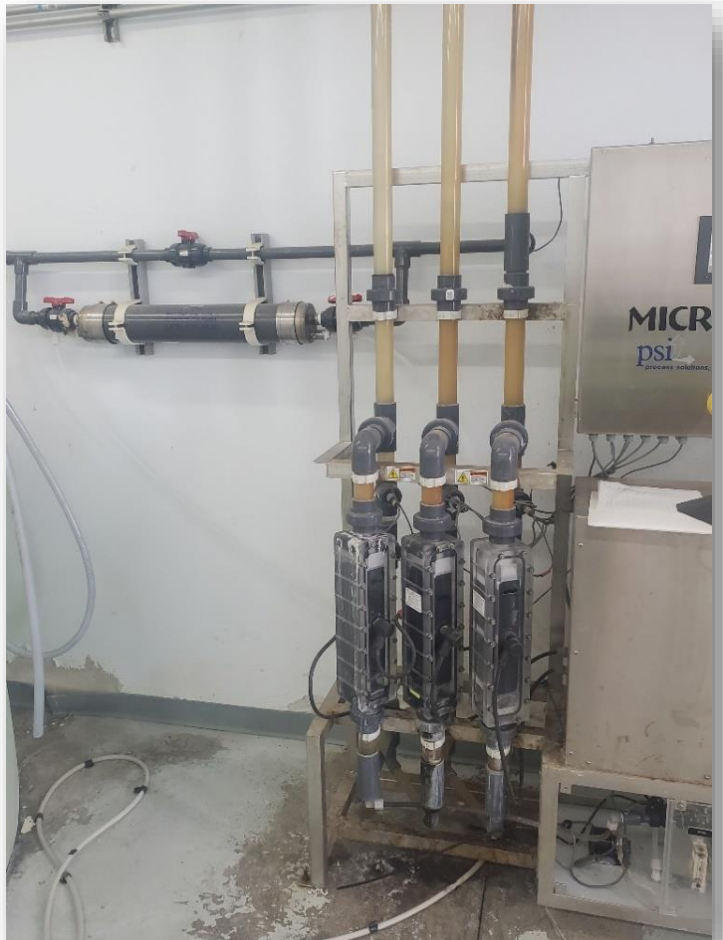
Chlorine Generator WWTP
