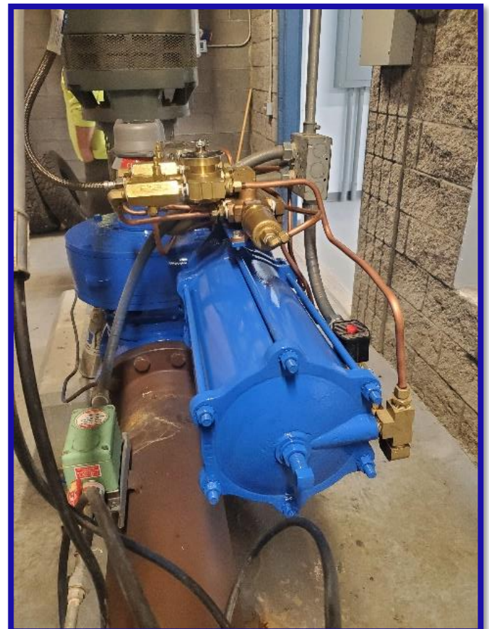
Skyline rebuilt Valve
