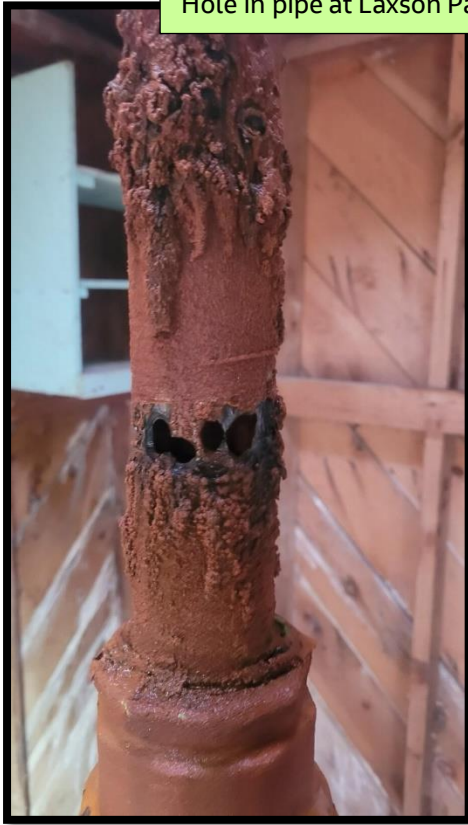
Hole in pipe at Laxson Park
