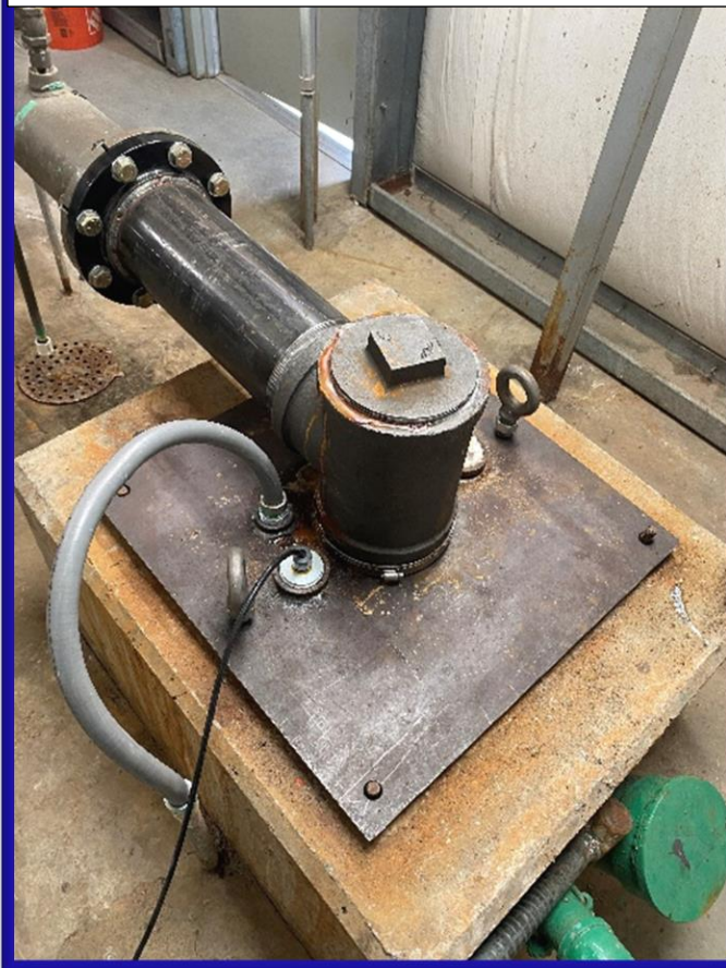
New Submersible pump installed at well #14
