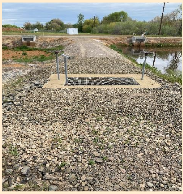
Erosion around recovery basin 1 and 2
