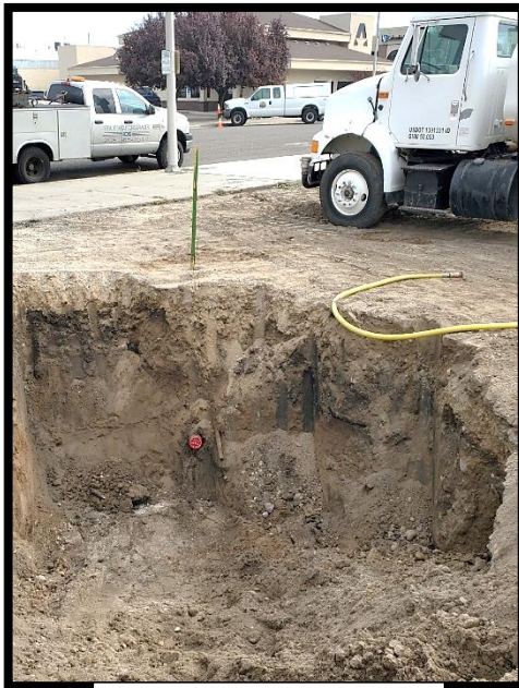
Abandoned Sewer Service
