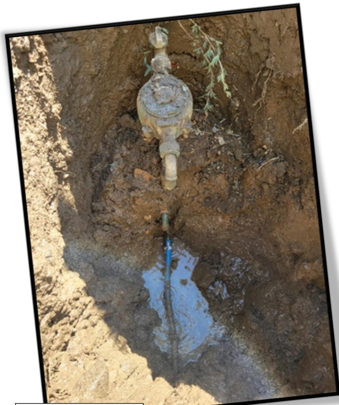
Leaking water service
