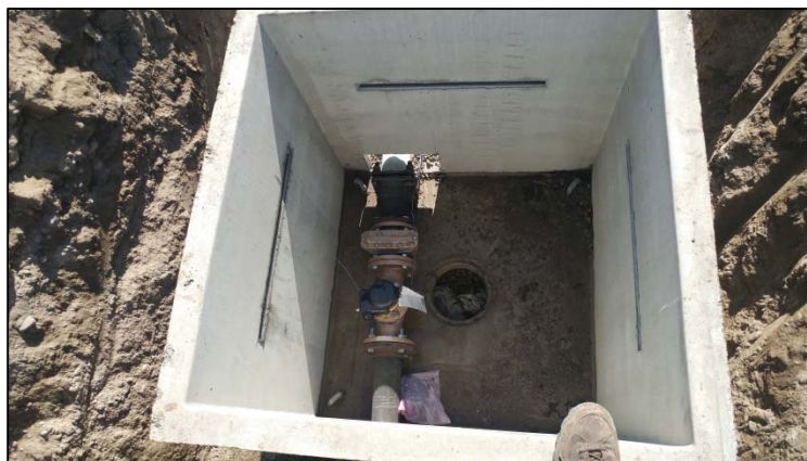
New 3-inch water meter for the Bureau of Land Management at the Ontario Municipal Airport.
