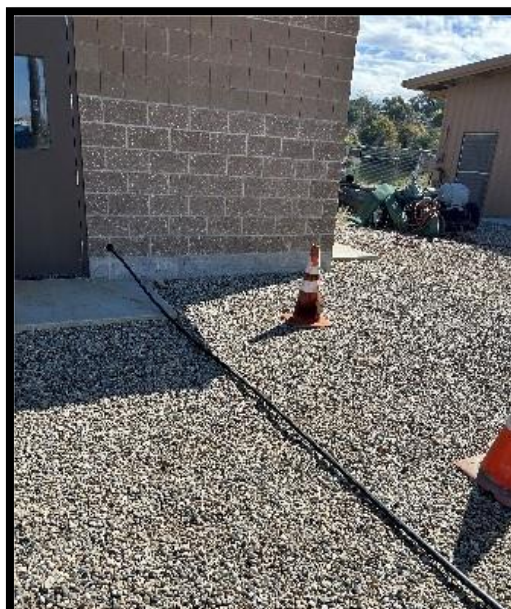
Temporary Chemical line installed for cleaning and maintenance.
