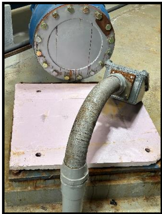
High Service Pump #1 removed for service & repair
