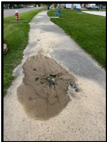
Leak in Laxson Park
