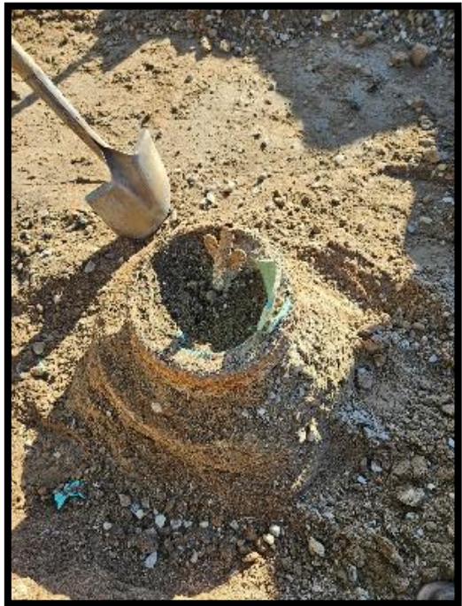
Lamp post for Sewer Main
