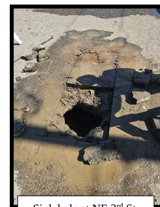
Sink hole at NE 3 rd St.
