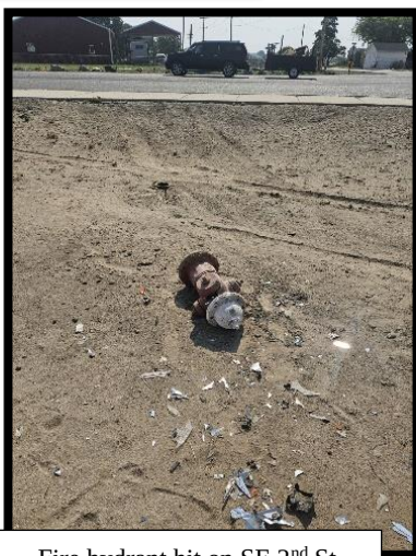
Fire hydrant hit on SE 2 nd St.
