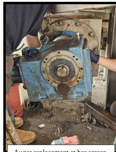
Auger replacement at bar screen.
