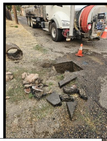
Water Service behind Library.
