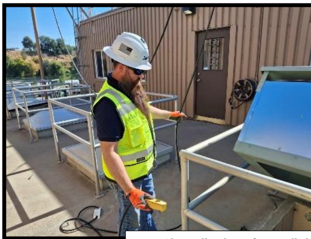
New Clearwell Exhaust fan installed.
