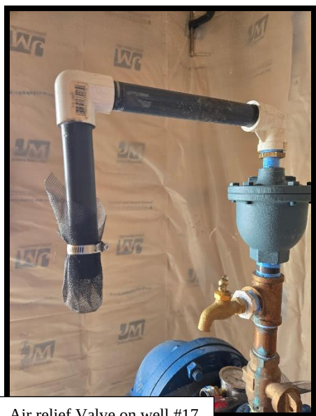
Air relief Valve on well #17
