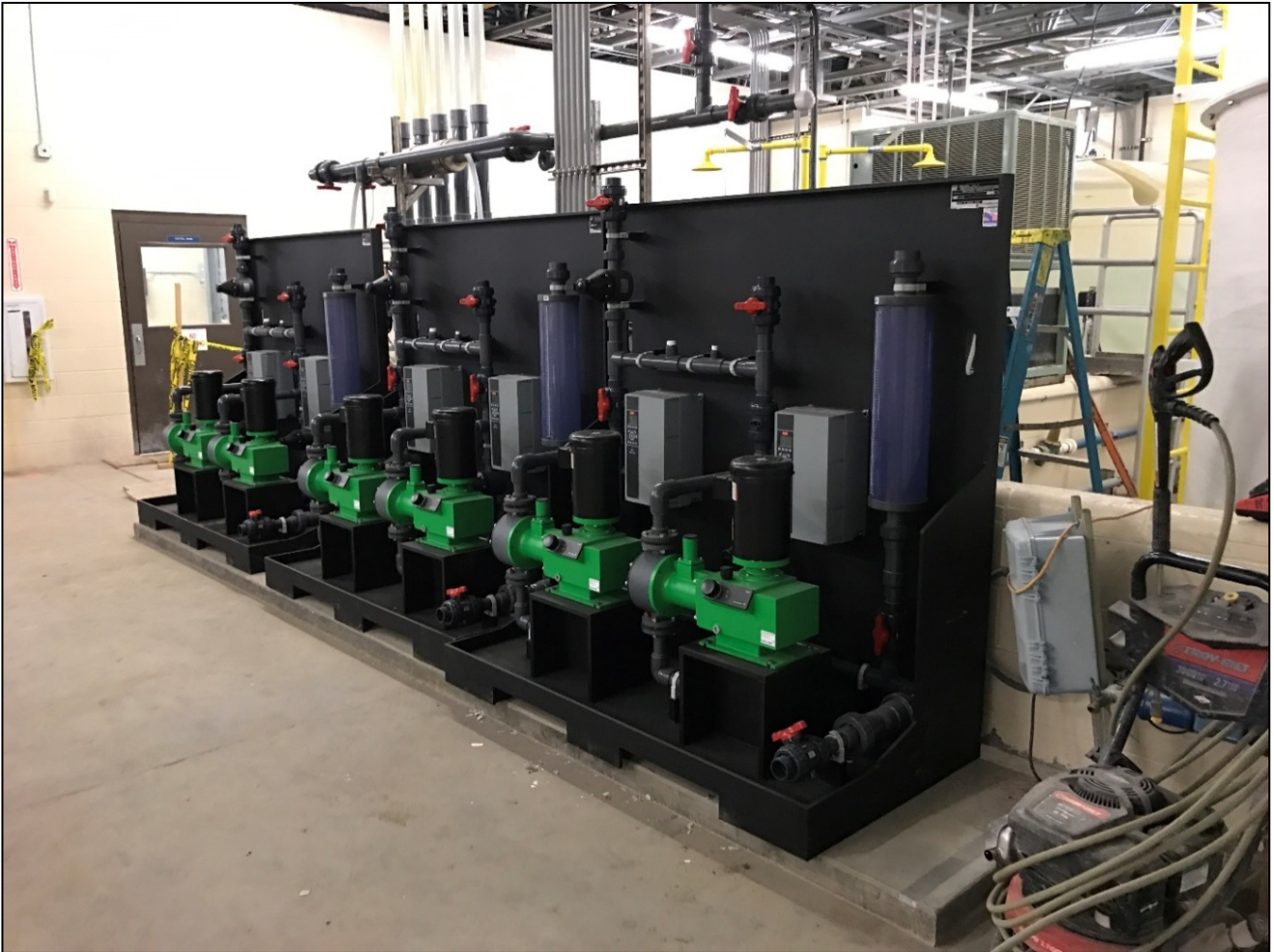
New chlorine chemical feed pumps at the Water Treatment Plant.
