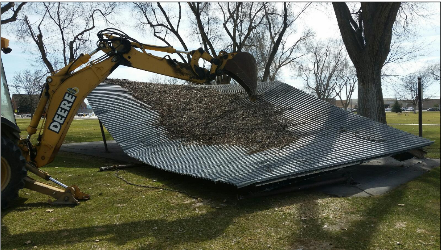
Tearing down the park pavilion at Lion's Park after the structural damage was discovered due to snow damage.
