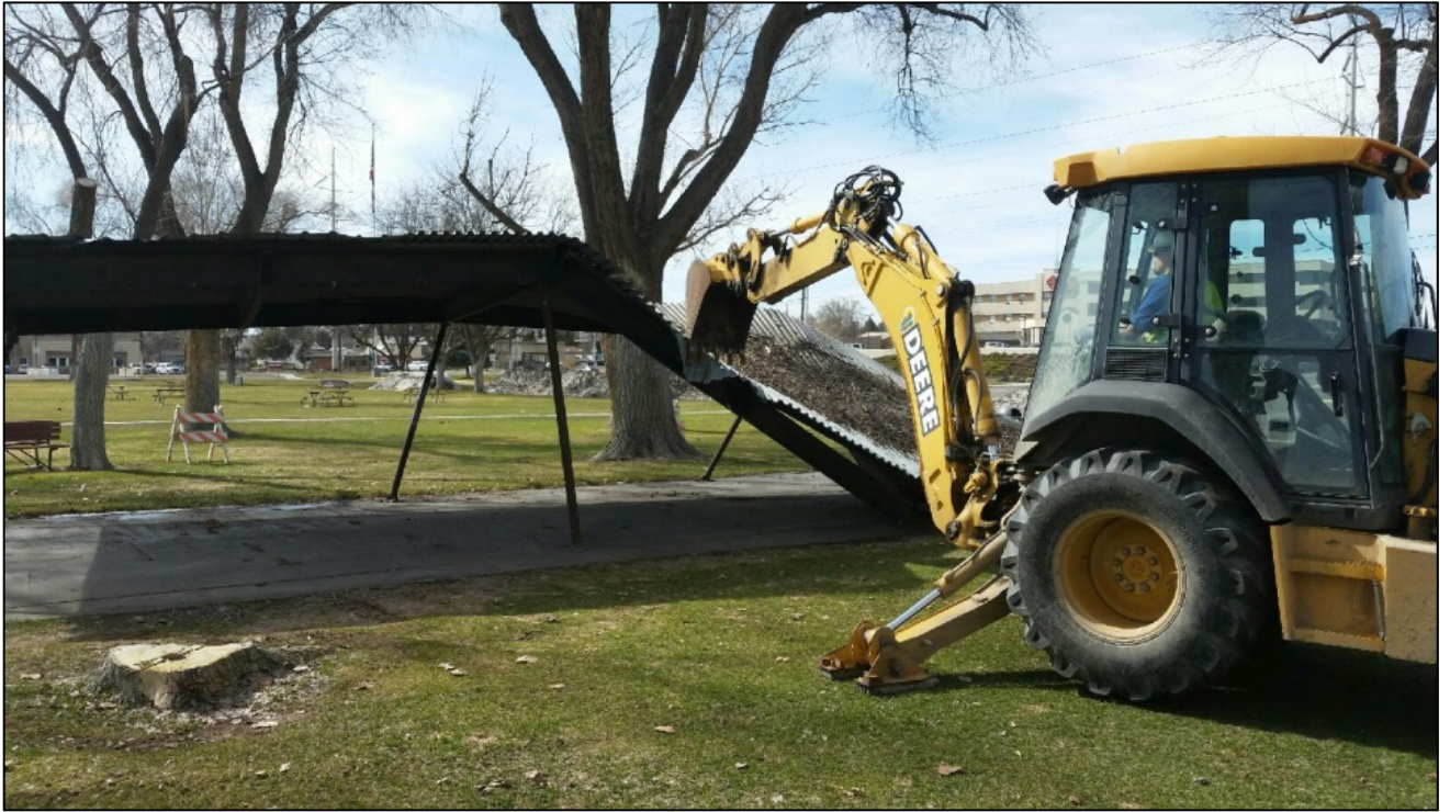
Removed a damaged pavilion shelter from Lion's Park. The heavy snow load broke a couple beams in the cover and could not be repaired.
