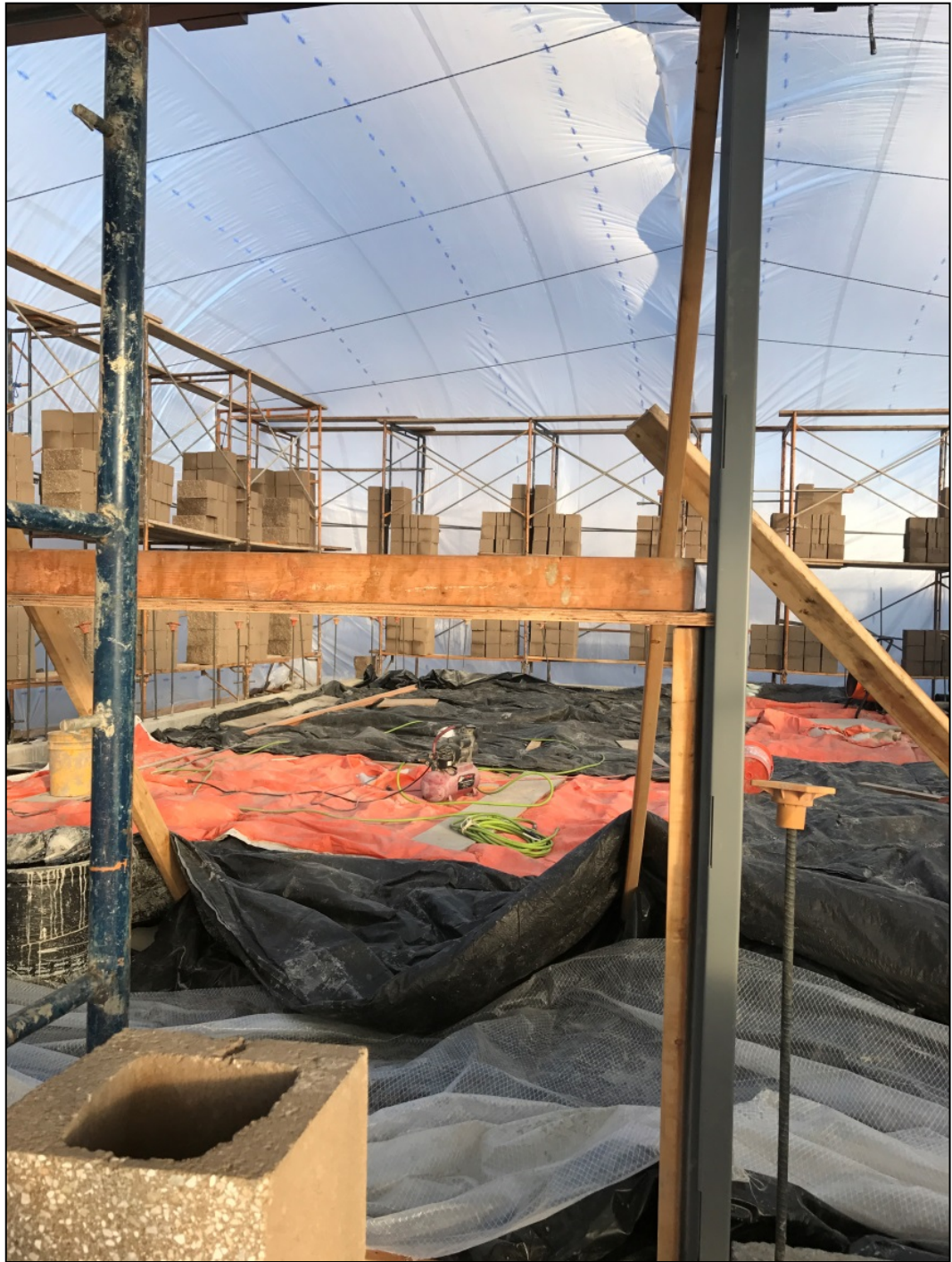
New chemical feed mixing building at the Water Treatment Plant.
