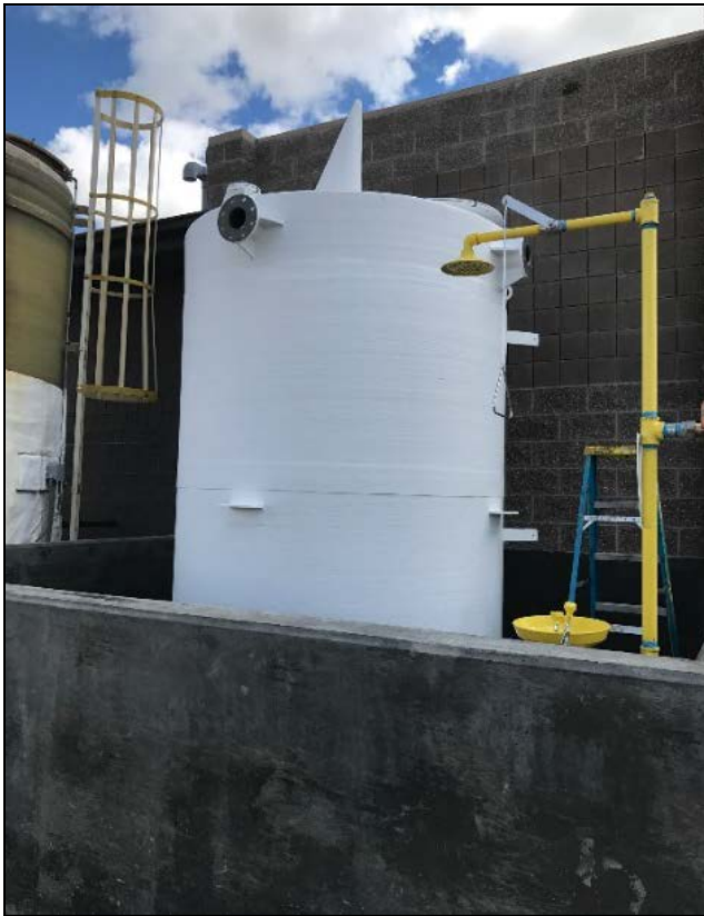
New caustic soda tank.
