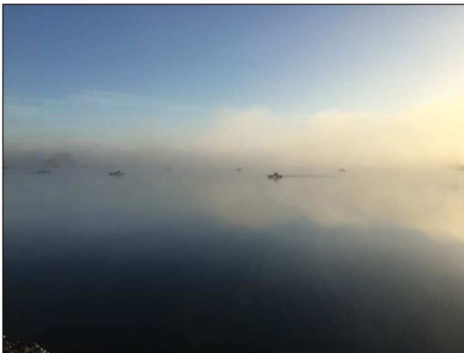
Aerators at the Wastewater Treatment Plant lagoons with a mist over the ponds on a foggy morning.
