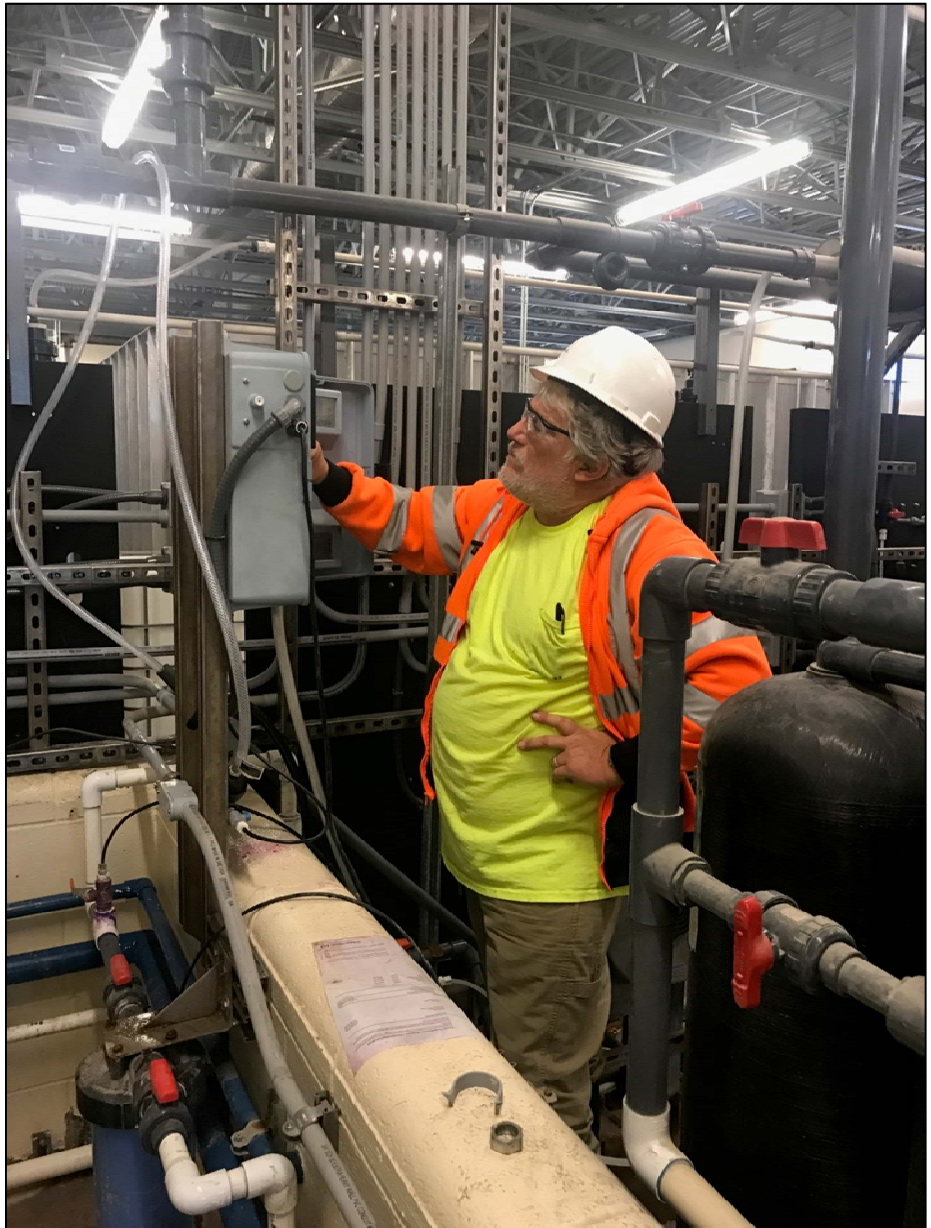
Water Treatment Plant employee calibrating the hardness indicator.
