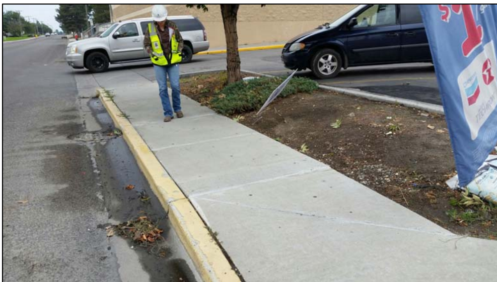
CH2M engineering technician inspects sidewalk pumping along Alameda Drive after several trip and fall complaints. Work to pump up low spots in the sidewalk eliminated uneven sidewalk panels.
